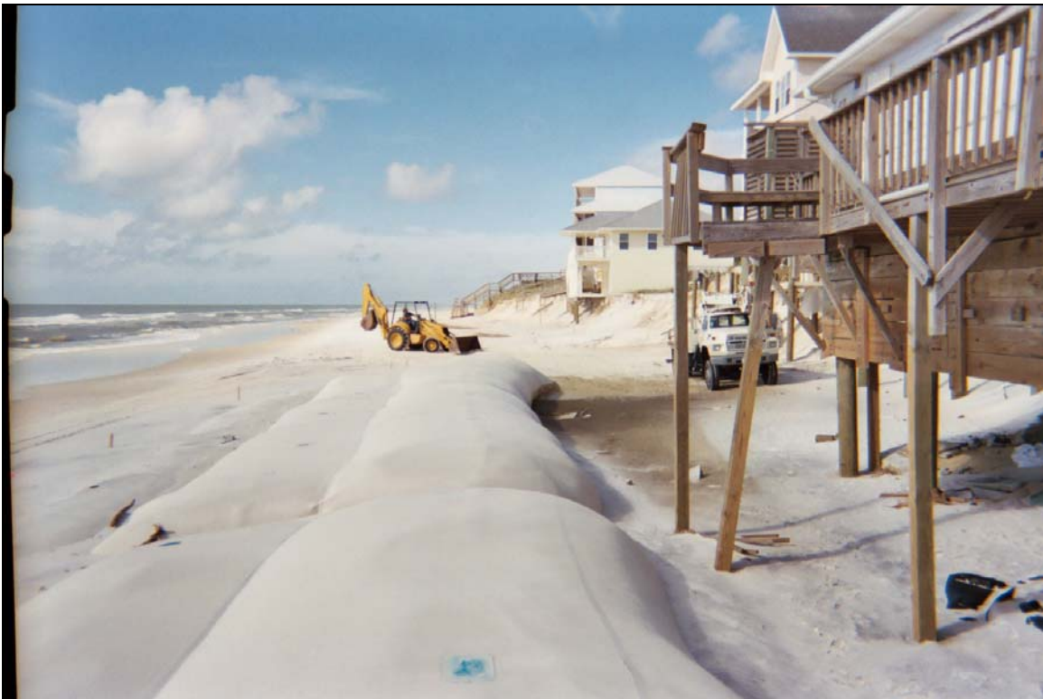
Figure 5. Post-storm damage showing scouring of dunes beneath structures as a direct result of wave action evidenced by Figure 4. Jeffrey R. Tabar, PBS&J (November, 2004)
