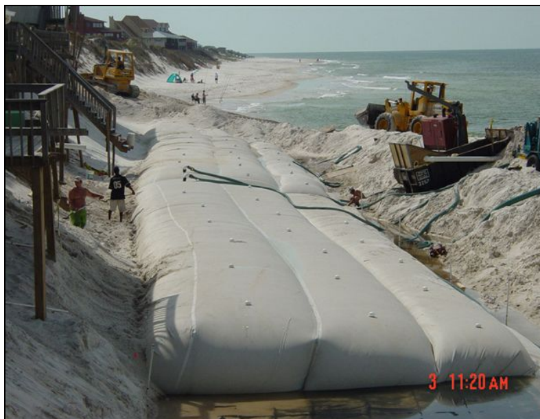
Figure 2. Installation of ProTecTube system showing the ProTecTube III's landward edge is flush with base of dune and the immediate vicinity of homes to be protected. Jay Sample, ACT Inc. (April, 2003)
